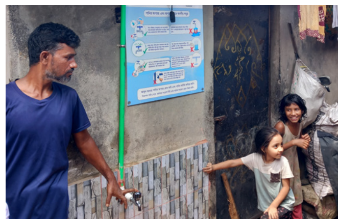
Image: Landlord stands proudly by a new water tap installed as part of WSUP project with support from The Coca-Cola Foundation. This communal water tap provides clean water from the municipal utility CWASA. The green pipe is connected to a water meter and payment is collected from the tenants to meet the regular bill. Previously residents had to pay approx. 700-100 taka a month for water from a private vendor, their share of the bill is now 200 taka a month. Credit: Emma Bakhle, Bangladesh, 2023
