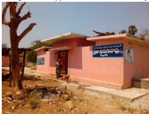
Image 13 No approach road for the facility
