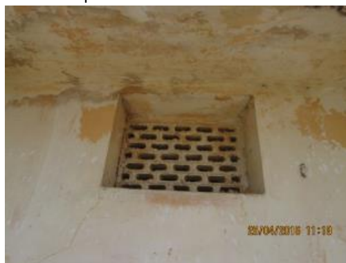
Image 27 No Ventilation and no exhaust fan in free to use community toilet facility, near Bheemunipatnam Beach
