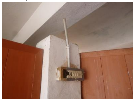
Image 26 Non-functional electric lighting in community toilet near Gavanapalem road (zone 7, ward 21)
