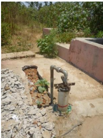
Image 15 A bore-well in community toilet of Santhinagar
