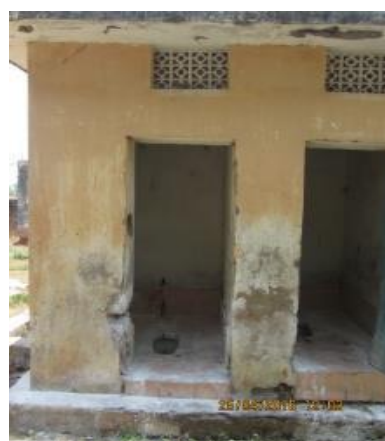
Image 32 No door in a CT at Lal Bahadur Shashtri Municipal Market (zone 8, ward 19)
