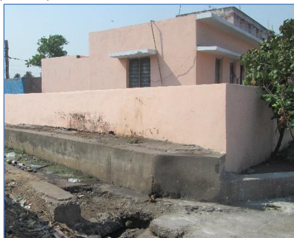
Image 18 A community toilet with waste water outlet into an open drain near Raythu bazaar, Bowdara road (ward 29)
