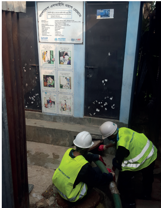
Image: Servicing a shared toilet in a low-income area of Chittagong. Credit: WSUP
